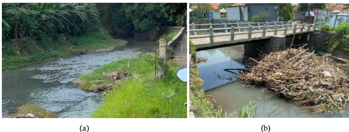
Figure 5. (a) Landslide on Existing Riverbanks (b) Waste Accumulation in the Existing River Source: Field Observation, 2024
