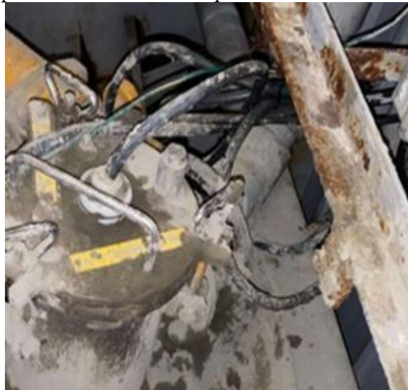
Figure 2. Pipe leak test confirming leakage points on flange and relief valve seat.
