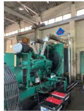
Gambar 2. Generator set 8 Mesin Diesel Cummins KTA38
